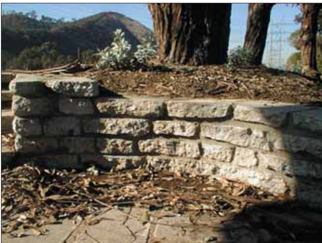
Figure 8.26 Broken concrete seatwall at Los Angeles Riverwalk at Los Feliz Boulevard
