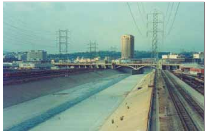
Figure 4.2 Entrenched trapezoidal condition at Fourth St. Bridge.
