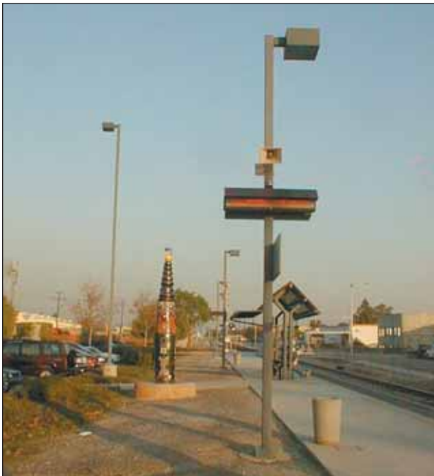
Figure 14.21 Shoebox luminaire at MetroLink Station, Pomona.
