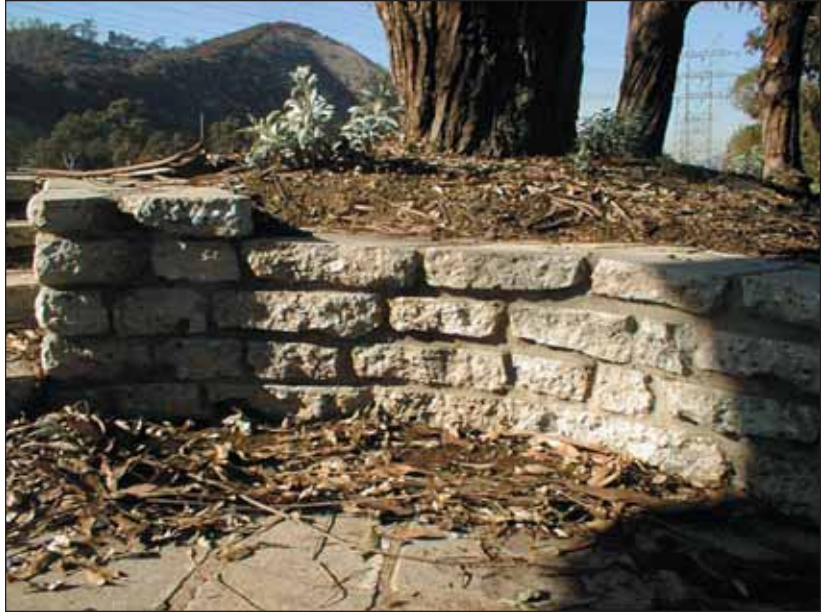
Figure 14.34 Broken concrete seatwall at Los Angeles Riverwalk at Los Feliz Boulevard, City of Los Angeles.
